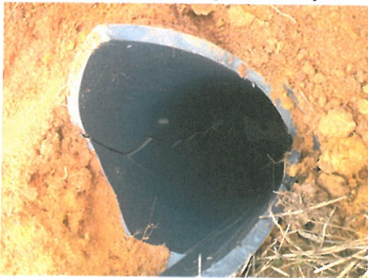
3 - Well shaft split vertically
