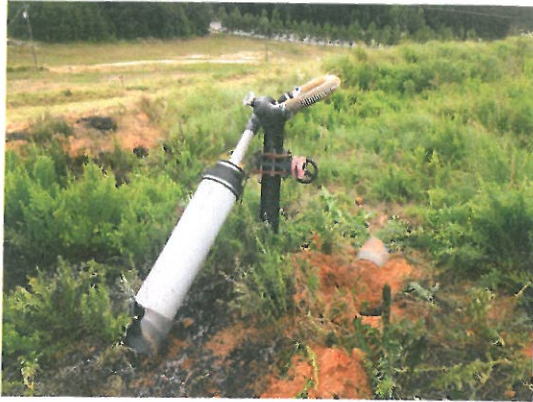
2 - Aboveground well head
