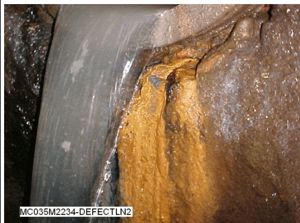
MC035M2234-DEFECTLN2 MH DEFECT 2
