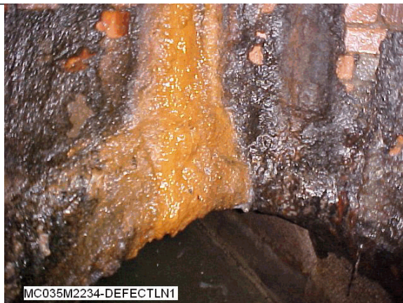
MC035M2234-DEFECTLN1 MH DEFECT 1
