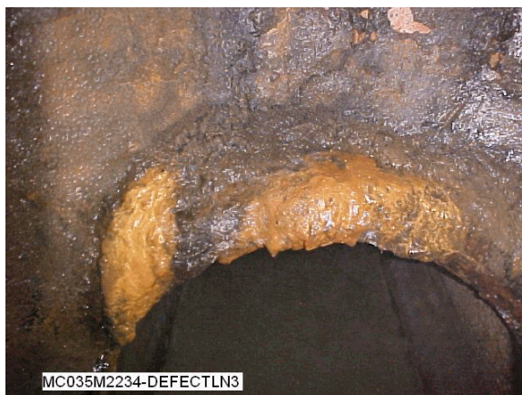
MC035M2234-DEFECTLN3 MH DEFECT 3
