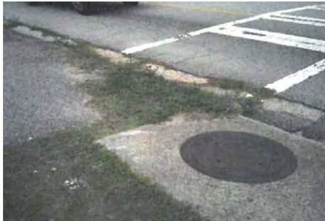
Figure 7-14. Missing Curb Ramp.
