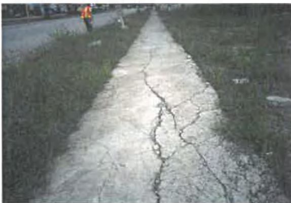
Figure 7-7. Cracked and Failing.
