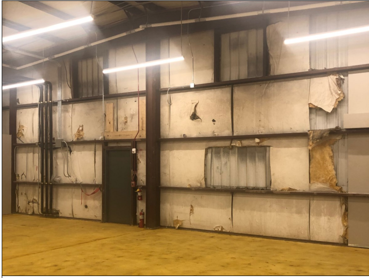
Damaged East Wall
