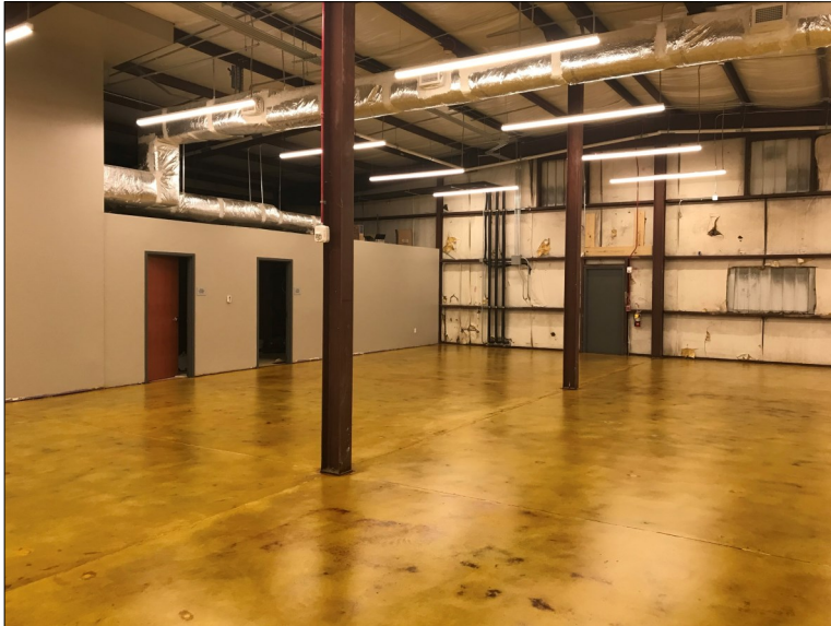
Sheetrock Wall and Damaged Wall
