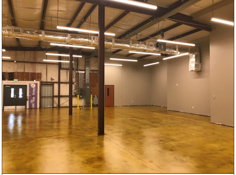
Stained Concrete Floor with Sheetrock Wall
