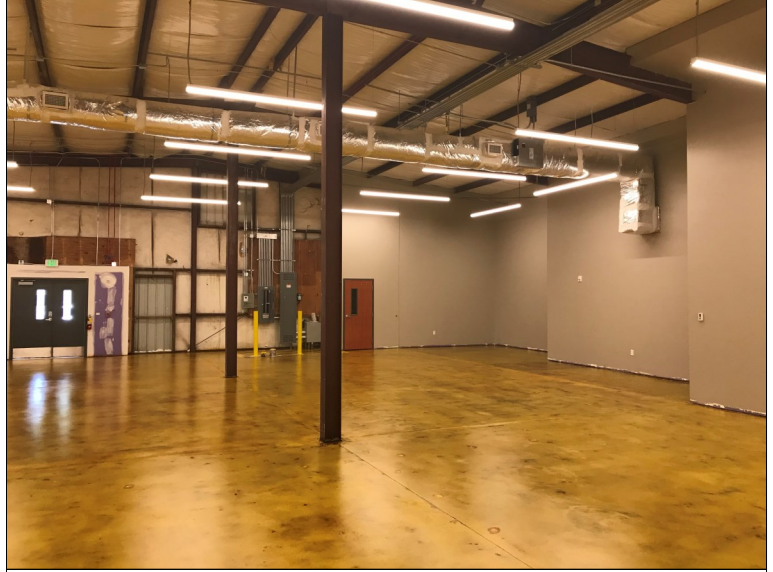
Stained Concrete Floor with Sheetrock Wall
