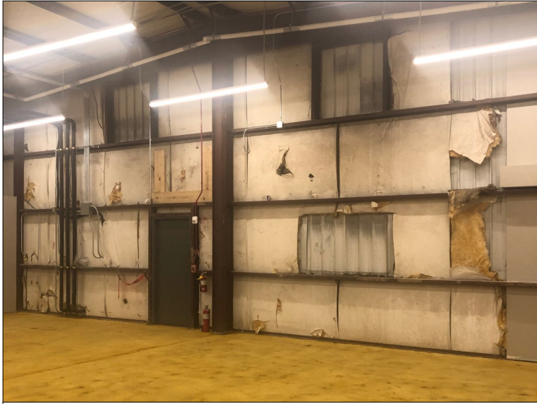
Damaged East Wall
