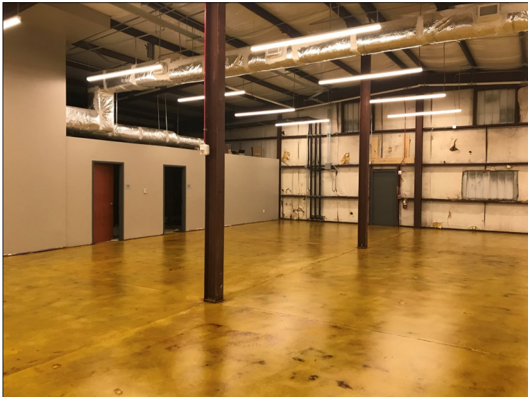
Sheetrock Wall and Damaged Wall
