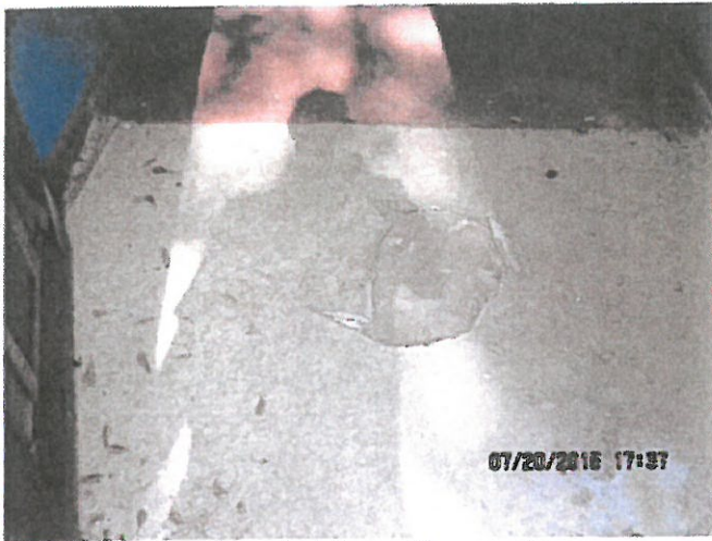
Photo 7 – Rock pattern vinyl floor with no mastic.
