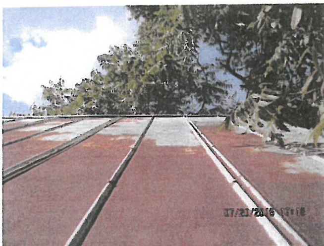
Photo 3 – Metal roof with no sealant/mastic.
