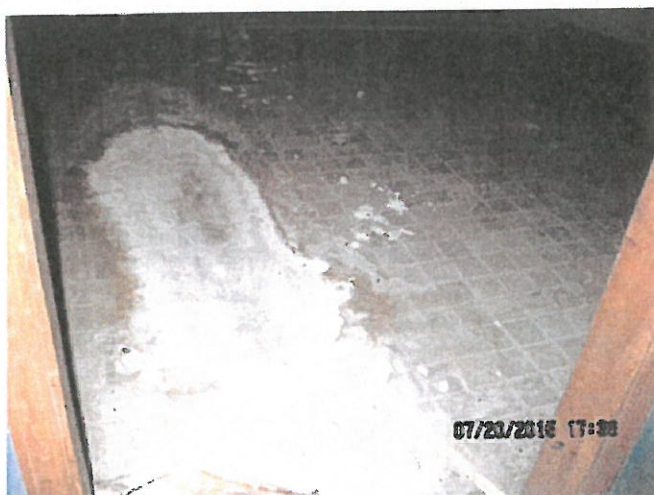
Photo 5 – Tan square pattern vinyl floor with no mastic.
