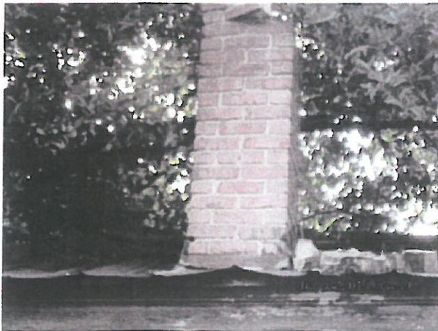
Photo 5 - Assumed chimney mastic.
